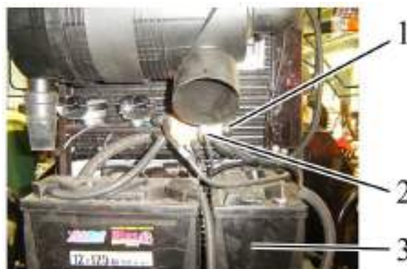
1 – button; 2 – AB manual disconnect switch; 3 – accumulator battery.
