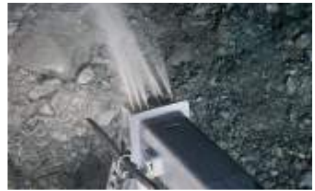
The water sprinkler system provides efficient dust control.
