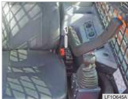
1) Cabin relay box
