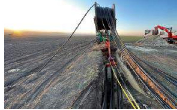
3 x 30 kV / 3 x 30 kV
